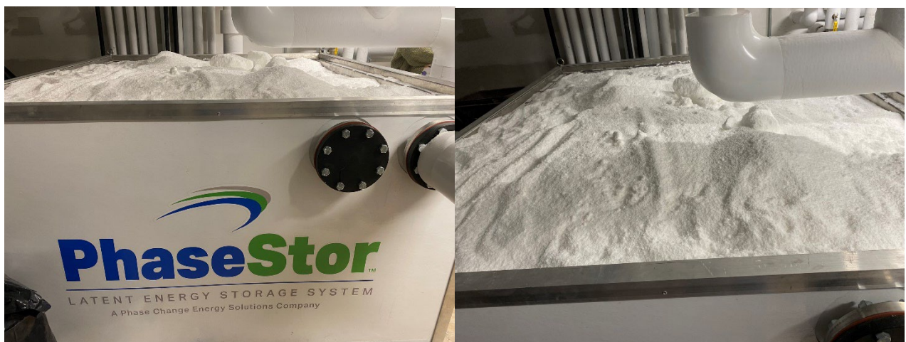
Image 4: Tank holding PCM after installation at Woodstock Fire-EMS building.
