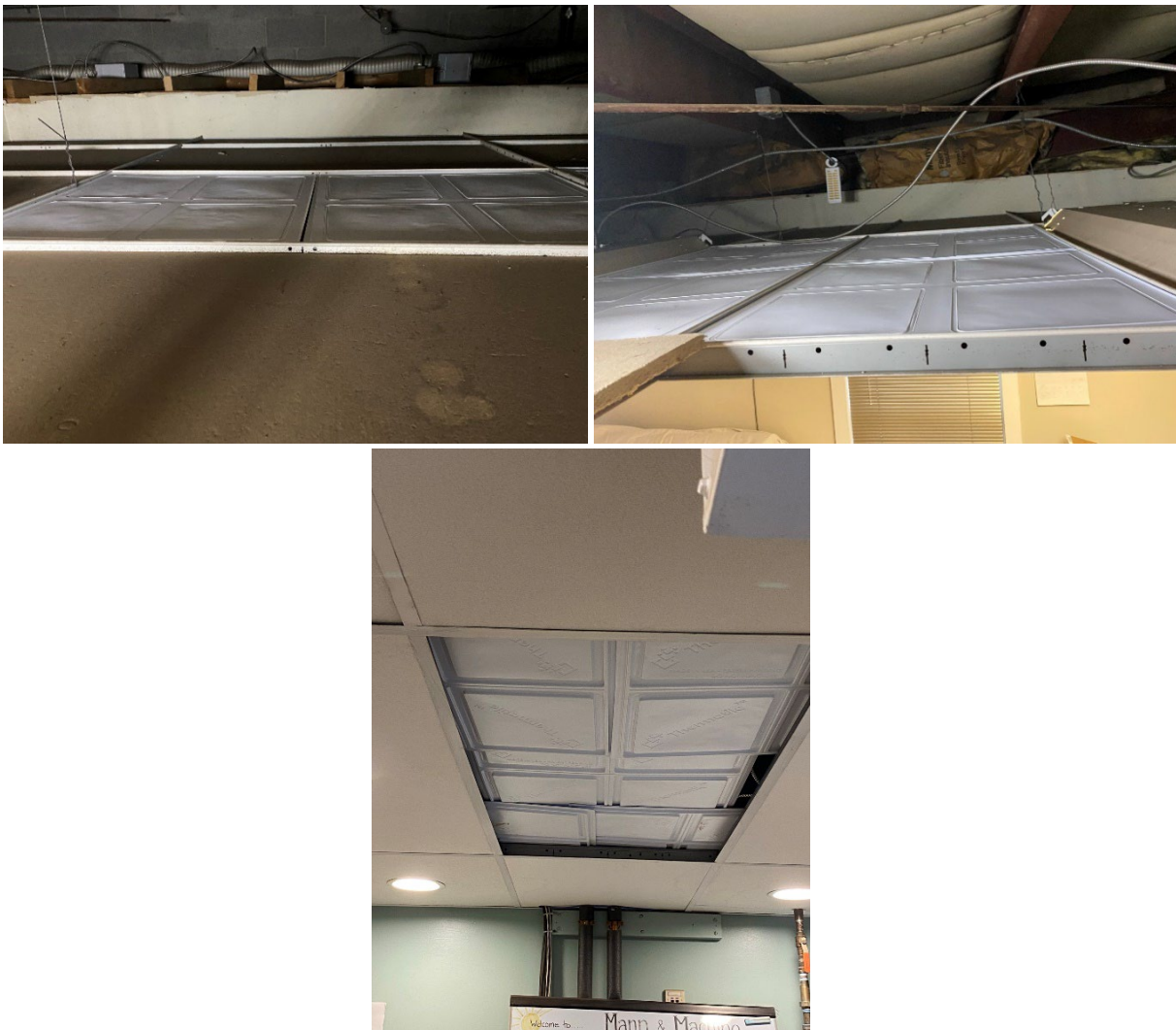
Image 2: Top left: PCM tiles installed above a drop ceiling tile on the first floor, Top right: PCM tiles installed above drop ceiling tiles on the second floor, Bottom: view of PCM tiles during installation process.
