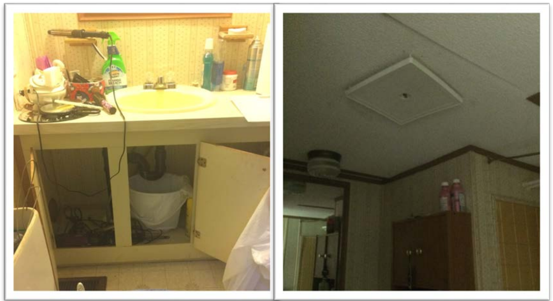
Figure 8. Pilot Home 2's bathroom, showing plumbing leak containment, cleaning supplies, and ventilation fan, prior to the energy-plus-health project.
