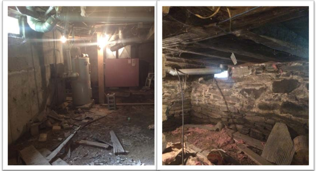
Figure 2. Pilot Home 1 basement conditions, prior to the project.
