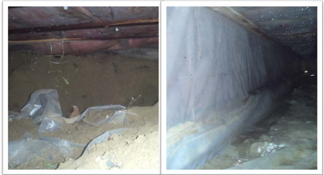
Figure 9. Crawlspace beneath the manufactured home, showing exposed plumbing and inadequate sealing and insulation.
