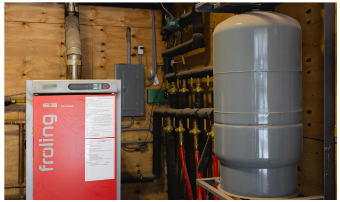
Two wood boilers (left) supply heat via a piped distribution system. The boilers can also "charge" three thermal storage tanks that can hold up to 1,800 gallons.
