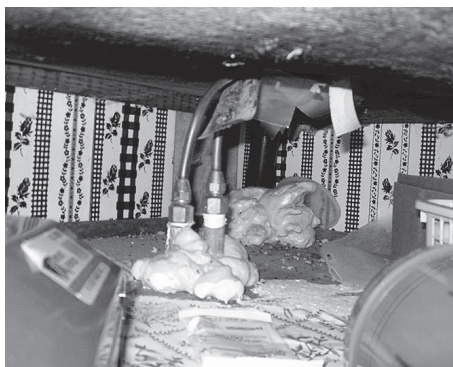
Small leak in cabinet sealed with foam
