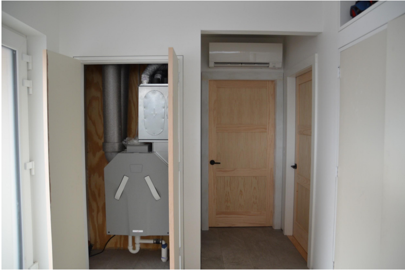
Heat pump above door in first floor entry
