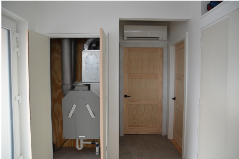
Ventilation Closet with Zehnder CA350 ERV
