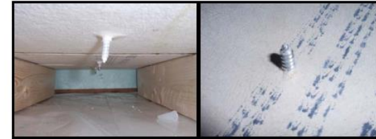
No leakage observed on screw bottoms
