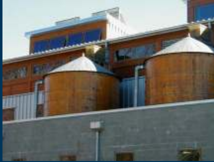
Rainwater cisterns at the Chesapeake Bay Foundation headquarters
