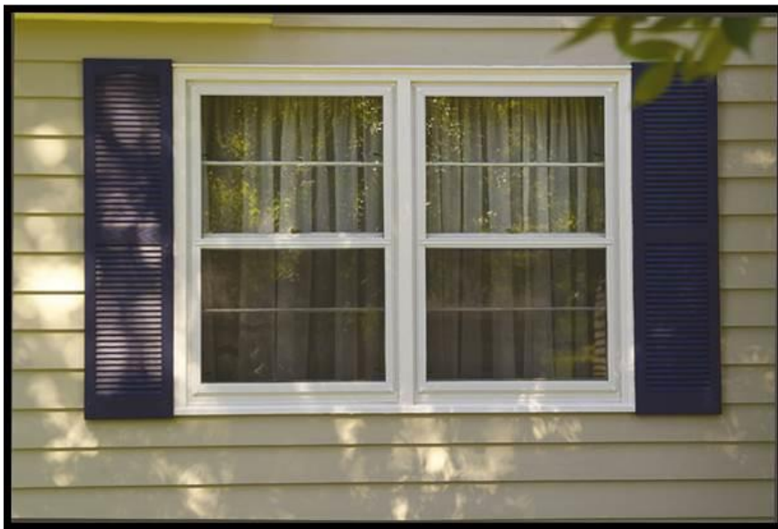
Figure 2. Modern Low-E storm window in place on a building.
